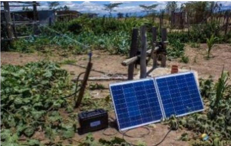
Solar powered water pump
